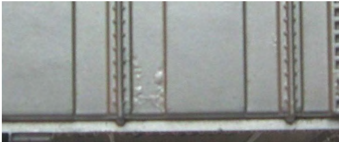
Figure #5 – Imperfections in painted finish.
